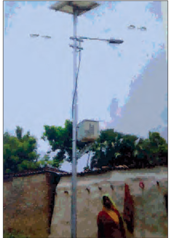
Solar Powered Street Light System provided in one of the backward villages of Ghazipur District (U.P.)
